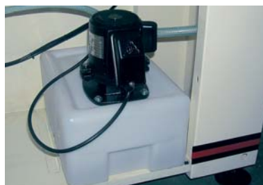
Complete coolant system
